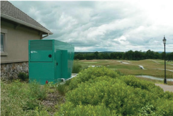
The 100 kW GGHH generator set, installed near the clubhouse, with the course in the distance.
